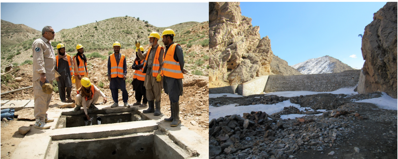
Figure 6 - Left. Cash for Work participants install a HDPE 2100 meters pipe scheme benefitting residents of Qafas and Mula Omar villages. Figure 7 - Right. The 5.1 square kilometre check dam constructed in Chakari village.
