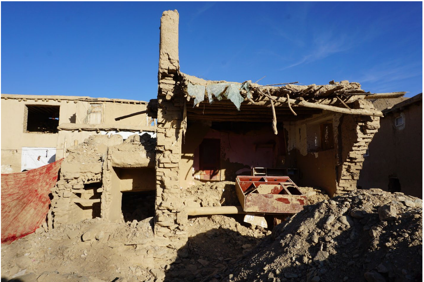
House destroyed in Takana Village, Maidan Wardak, Afghanistan.
